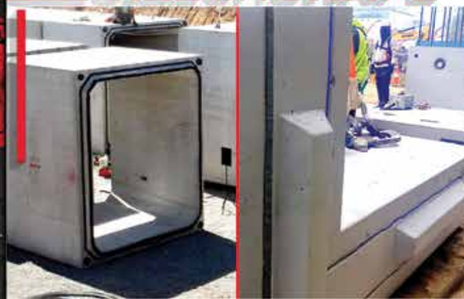
1 MILLION GALLON WATERTIGHT STORMWATER DETENTION SYSTEM
