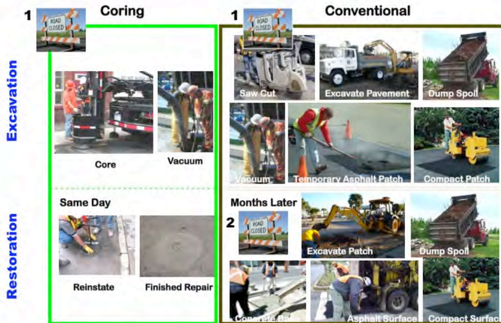
Figure 2: Comparison of equipment and timelines in coring and reinstatement and conventional excavation technology that affects the Carbon Footprint. Graphic courtesy of Utilicor Technologies Inc.
