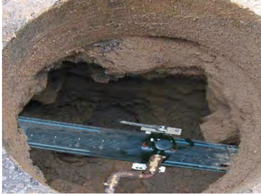
Figure 11: New HDPE pipe (black) connected to lateral through electrofused tee and copper connector (AwwaRF 2007)
