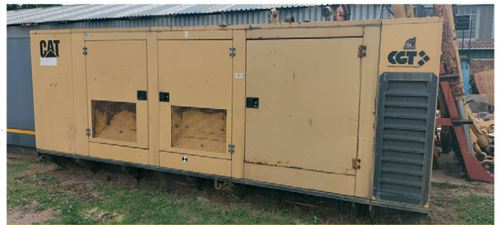
KVA 450-500 C18 CAT ENGINE
