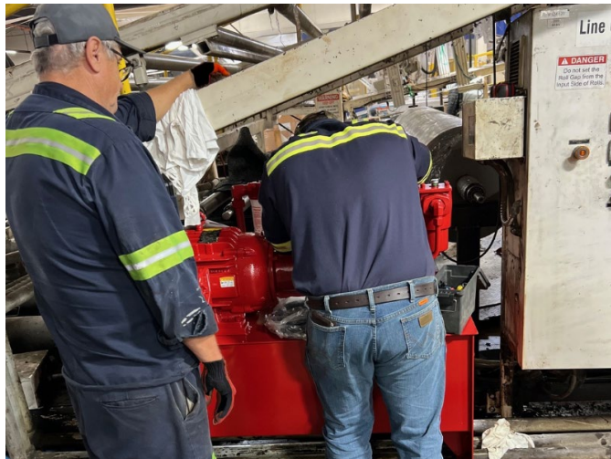
Figure 1: Despite a time crunch, our team managed to complete this job for the customer in just 14 days.
